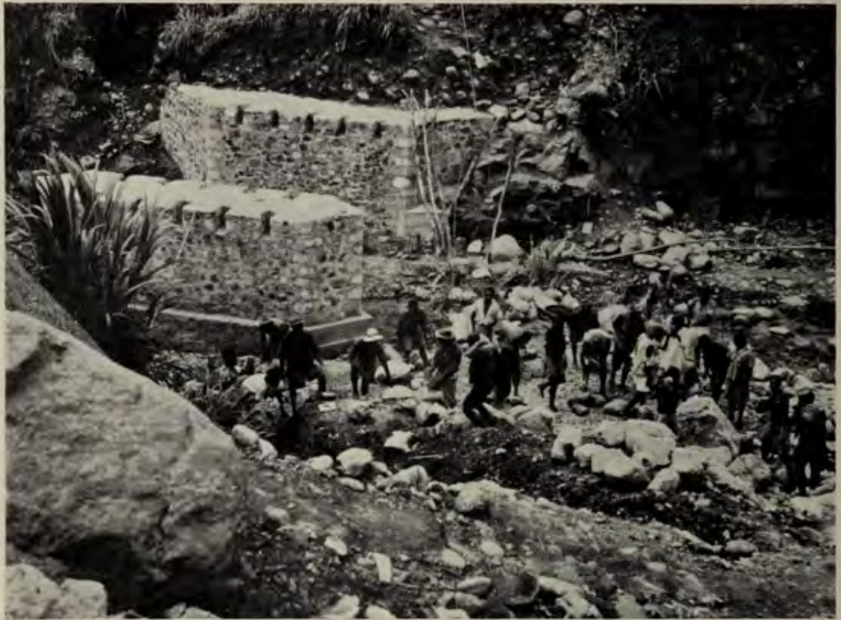
Voluntary labourers building roads and bridges in the mountainous country of BAFUT
